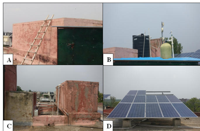
Fig. 1 Reservoirs: A – Inlet tank supplying groundwater to RO plant; B – Outlet containing purified water from RO plant; C – Wastewater storing tank of RO plant; D – Solar Panel
